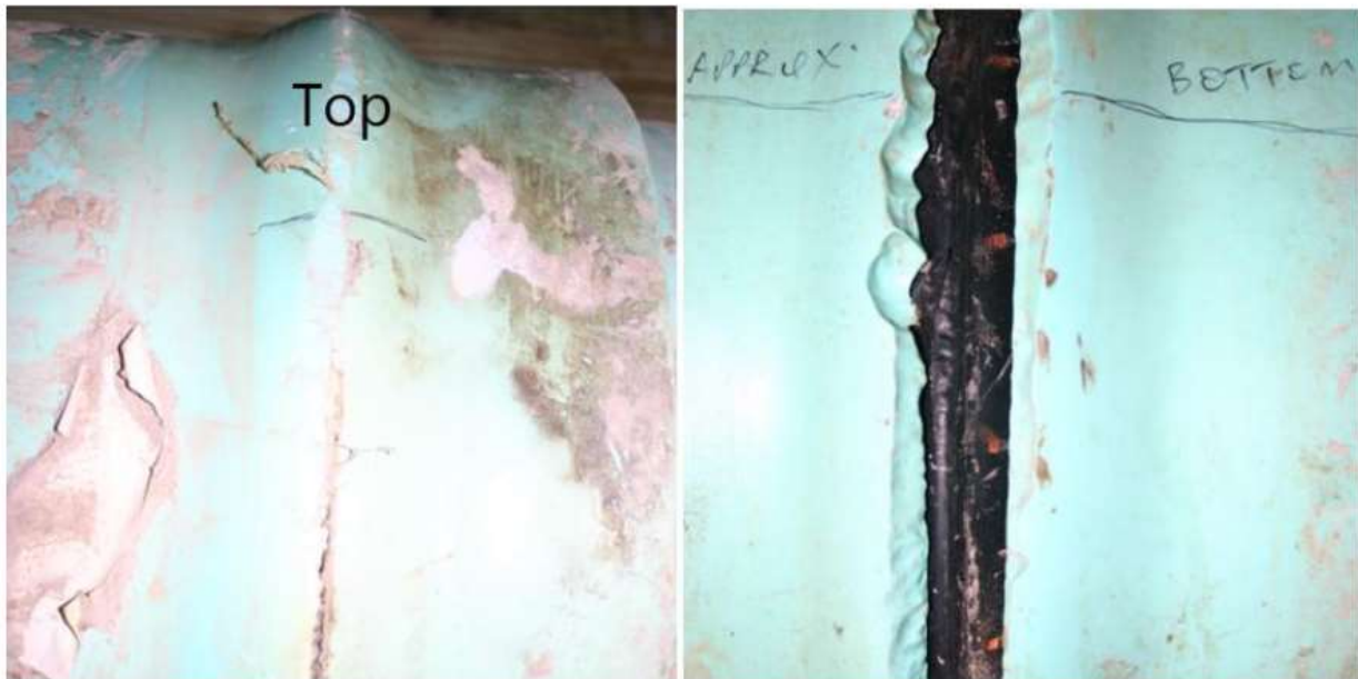
Figure 5. Photographs showing the top and bottom locations of the fracture in the bell of the pipe as received. Notice the extensive erosion of the fracture surface in the photo on the right. The erosion was caused by the rapid flow of water through the crack over an extended period of time. The gasket/seal is visible through the crack on the photograph on the right.
