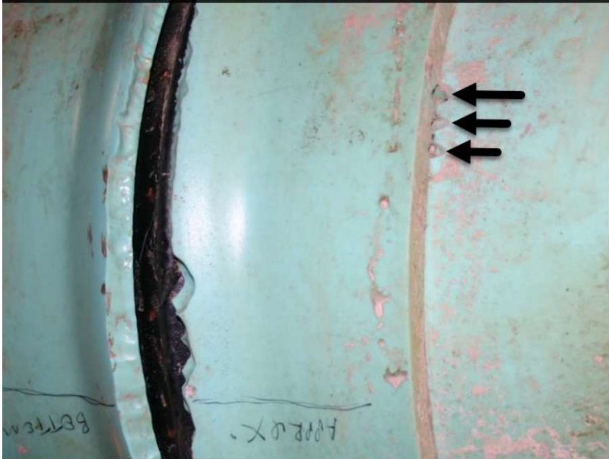
Figure 3. Black arrows indicate erosion caused by the exit of water from the joint before the circumferential crack formed in the gasket trough.
